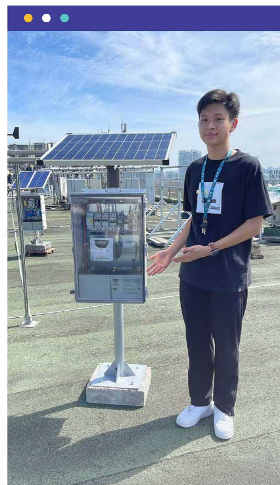
SOLAR PV SET UP
